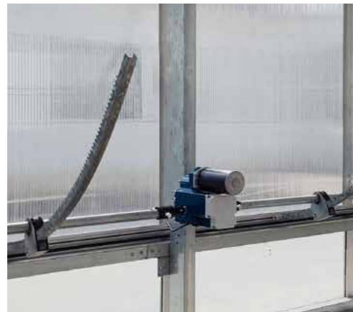
Rack and Pinion Ventilation
