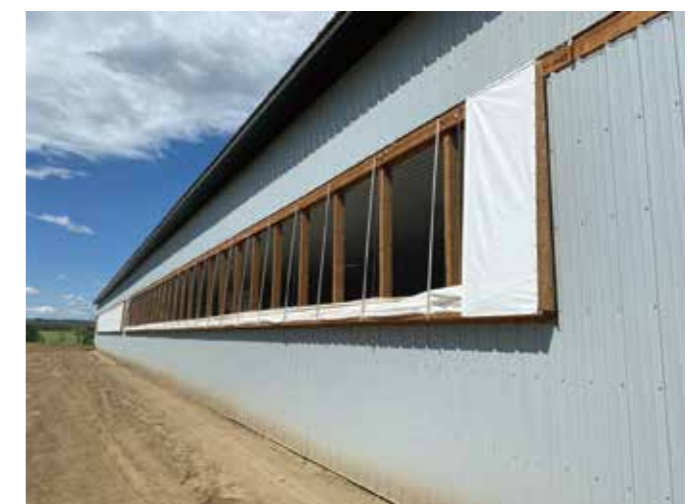
Top down Curtain Ventilation
