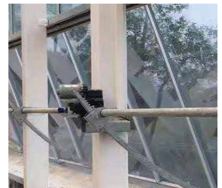
Rack and Pinion Ventilation
