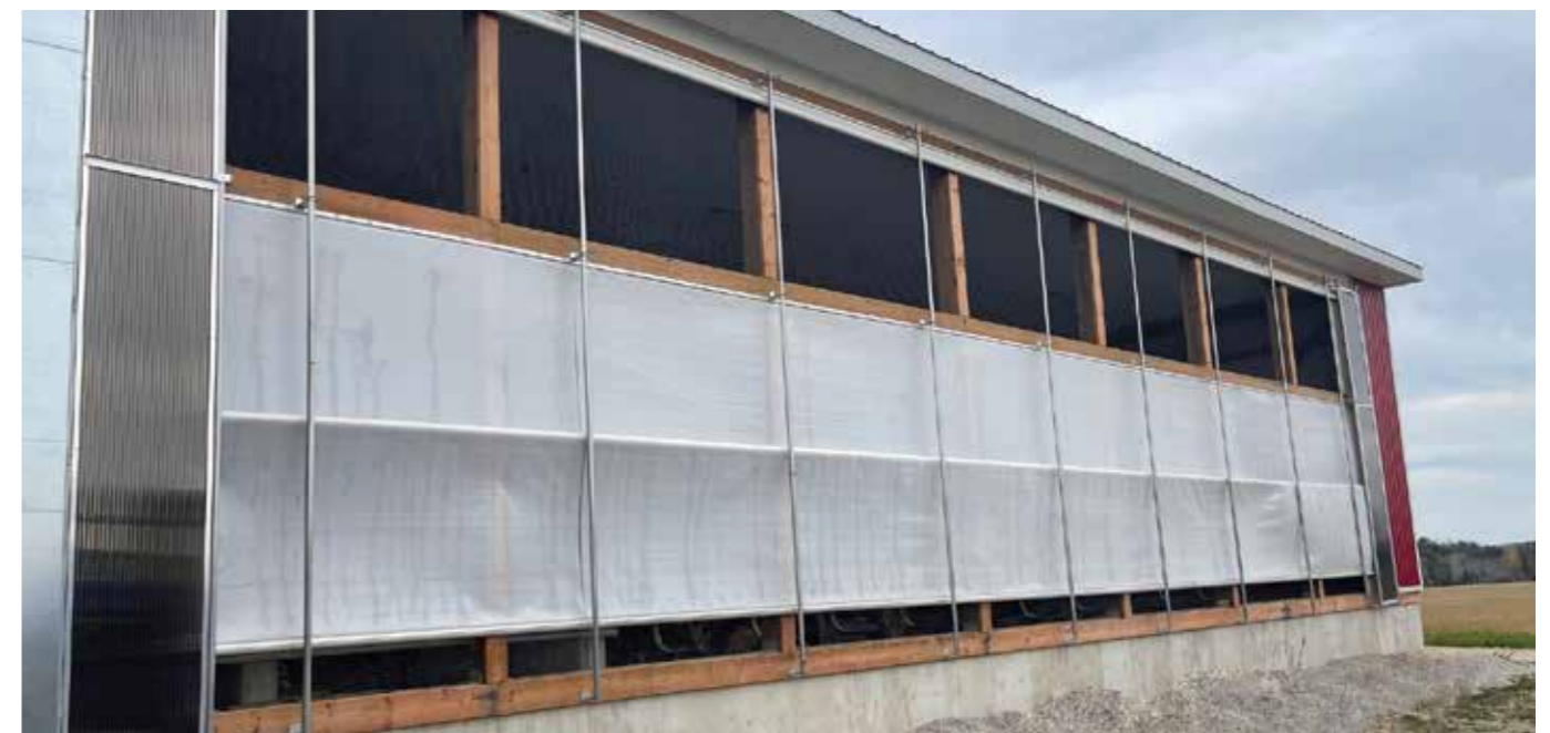
Curtain Vent system
