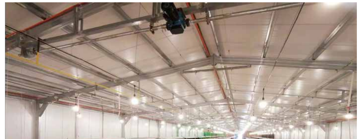
Feeding line Hoisting System
