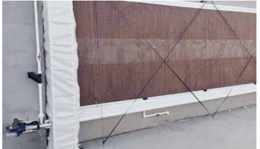
Roll over Curtain Ventilation
